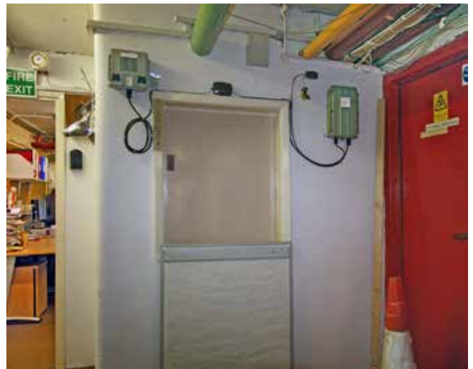
WB1401 receiver (right) and speaker in the Operations Room.
